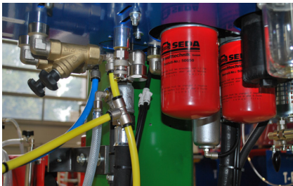
Inline filter system
